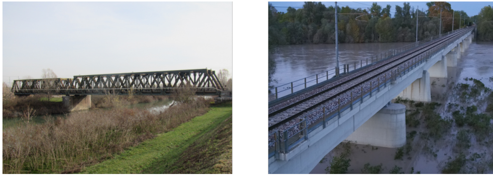
Figure 2. Photos of the railway bridges object of this study. On the left, the Warren truss bridge; on the right, the CACP bridge.
