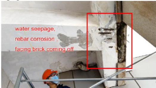
Figure 1. Water seepage, rebar corrosion.
